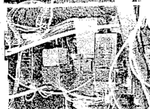
5.71 Relay panel unit location under fascia
