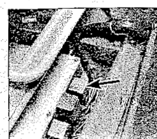
6C.95 Fuel pump relay location (arrowed) under right-hand front seat
